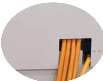
Aperture in lower edge of door allows five generator cables to exit the cabinet with the door padlocked shut.
